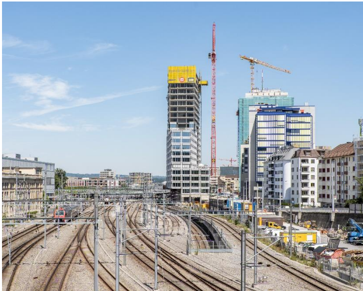
Caption: The facade installation work is already in full swing and the expansion work is also in progress at full speed. Copyright © Roman Keller, Zürich
