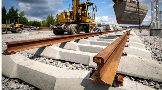
Railway Engineering Transfer point Bytom
